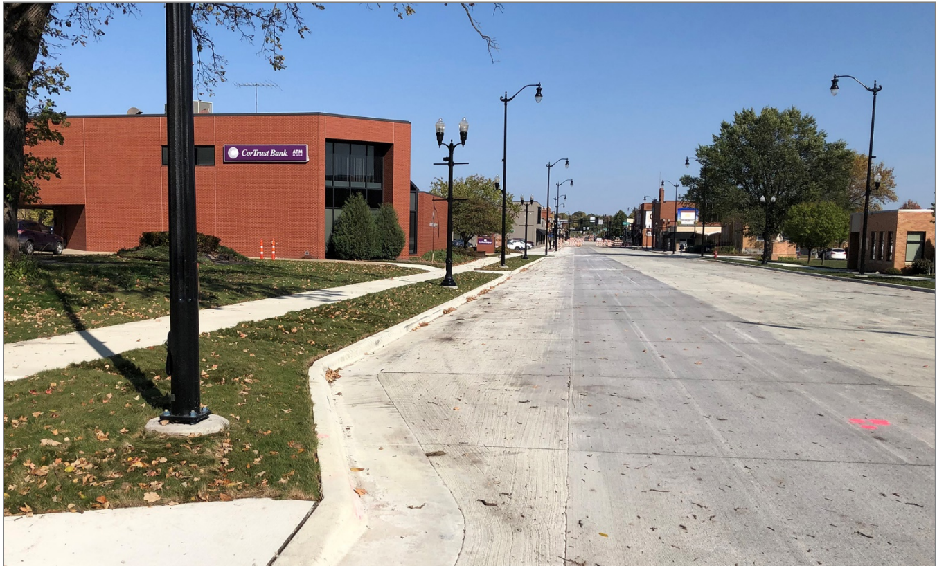
Photo above: looking north from 4 th Avenue, lighting systems and grass boulevards have been installed on Hwy 15/Main Street.
