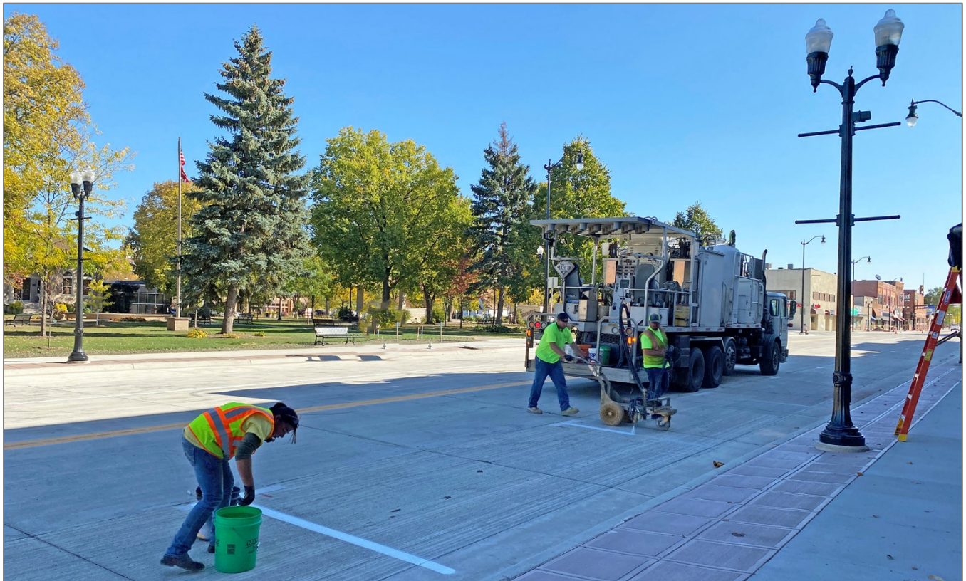
Photo above: crews paint parking stripes along Hwy 15 between Washington Avenue and 1 st Avenue South.
