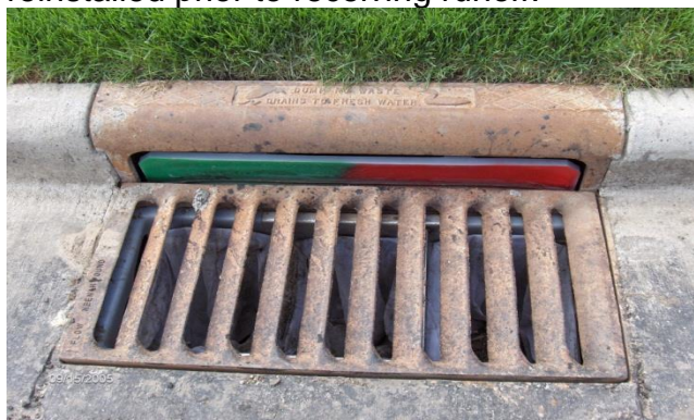
Inlet protection installed in a new subdivision. The purpose is to capture any sediments that are in the curb line while still allowing stormwater to drain.
