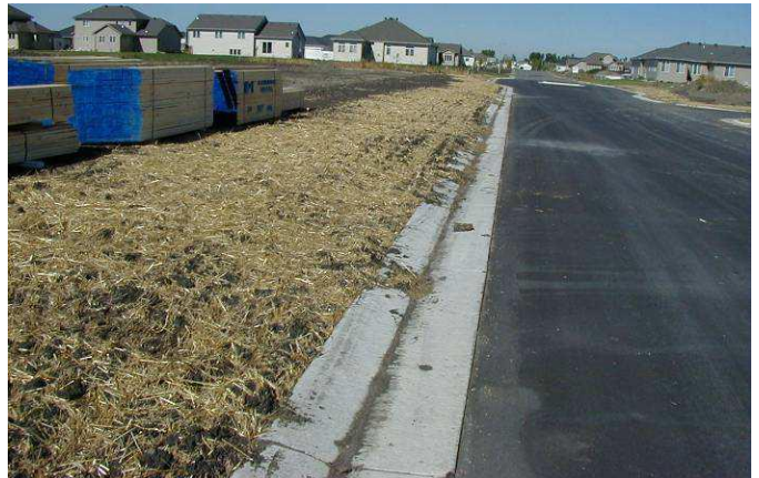
Boulevard recently seeded with disk anchored straw mulch applied to prevent sediments from entering the curb line.
